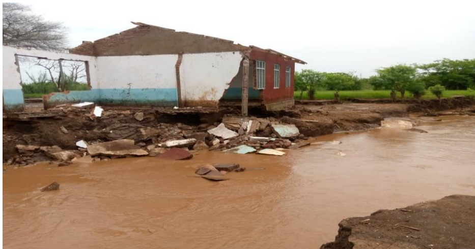
Photo 1: A Primary School in Mambegwa Village (Msowero Ward) Completely Demolished by Floods in February 2022 (Used with permission from the Village Chairperson).
